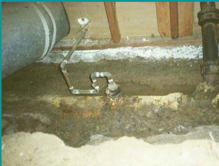
Water softener regeneration discharge to soil pipe
